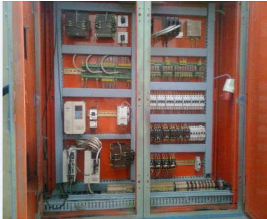
Fig.3 PLC based control panel for EPG
