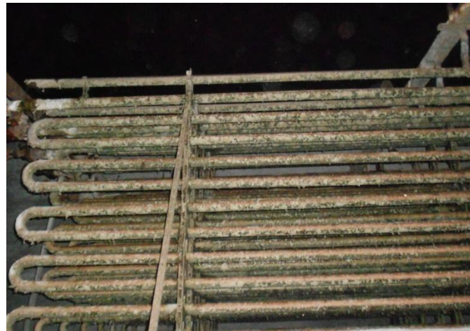
Fig. 2 before removing the corrosion and algae from the condenser tube
