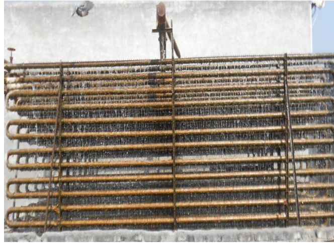
Fig. 3 after removing the corrosion and algae from the condenser tube
