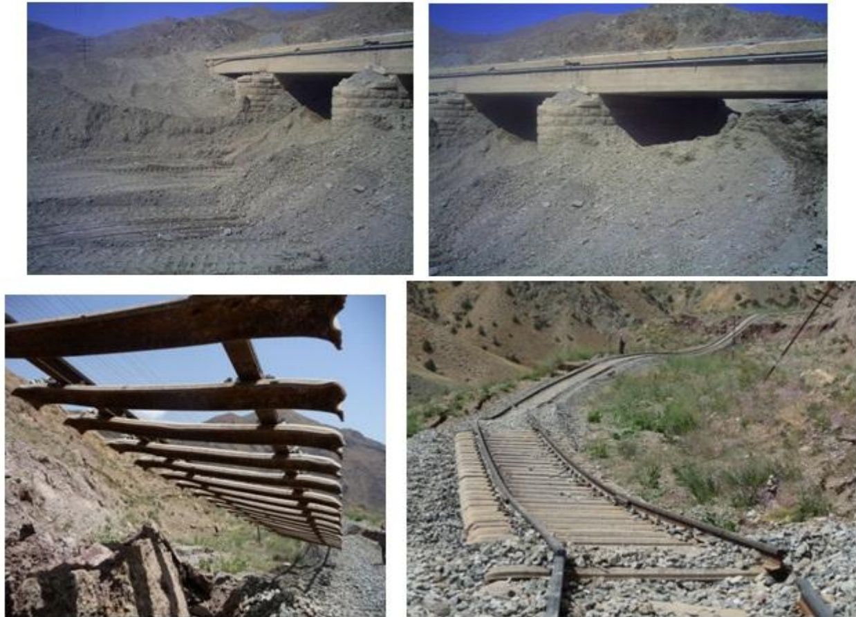
Figure 5-landslides on the road
