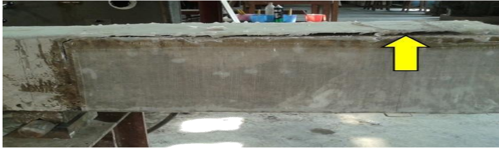
Figure 3.20 Debonding failure of FRP
