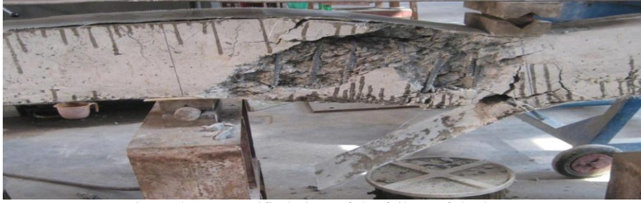
Figure 3.16 Magnified view of the failure of the beam
