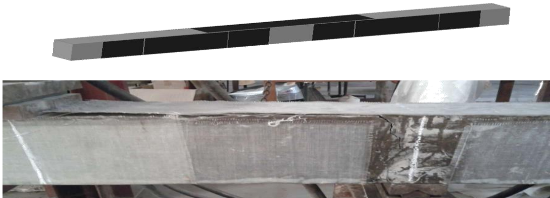
Figure 3.26 Debonding of FRP and cracking pattern above central support of the beam
