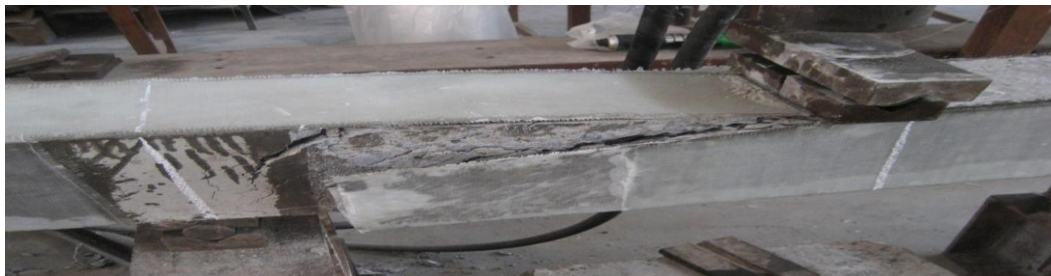
Figure 3.42 Shear crack in the left span
