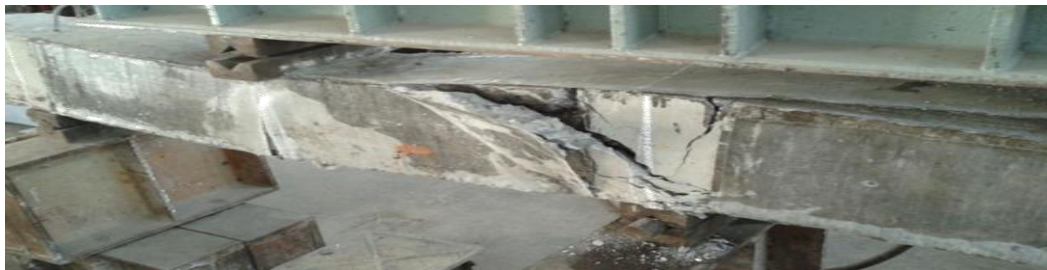
Figure 3.18 Ultimate failure of beam by debonding of FRP with concrete cover
