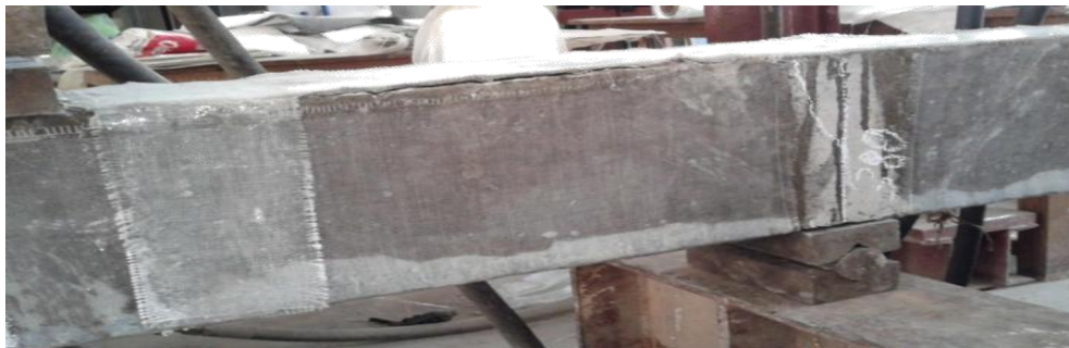
Figure 3.22 Crack pattern after initial loading
