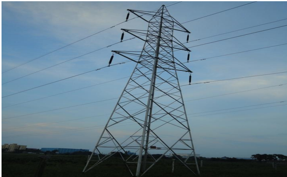
Figure 1: 132 KV GNT-TDK DC TOWER
