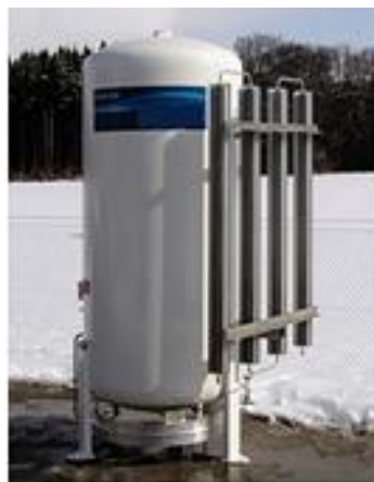
Figure 3 : Storage tank of LO 2
