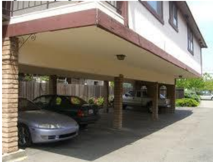
Fig-1: Example of a soft storey at the ground floor.
