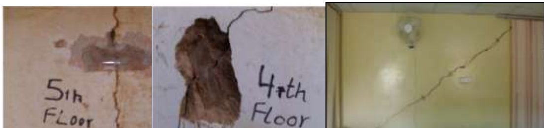
Figure 4 shows pictures of the cracks that have occurred in the building at different floors (the eastern and south-eastern part of the building)
