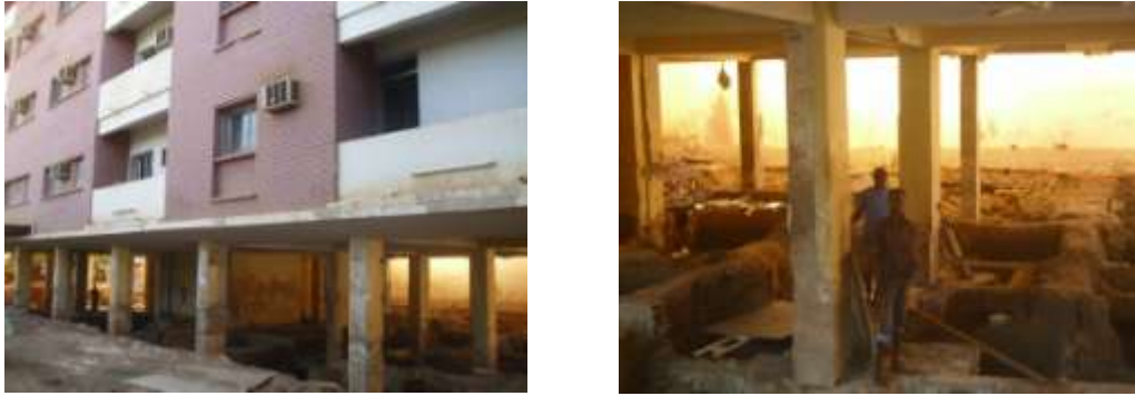
Figure 8. Pictures of the building during a digging to see the foundation type and water sources under building
