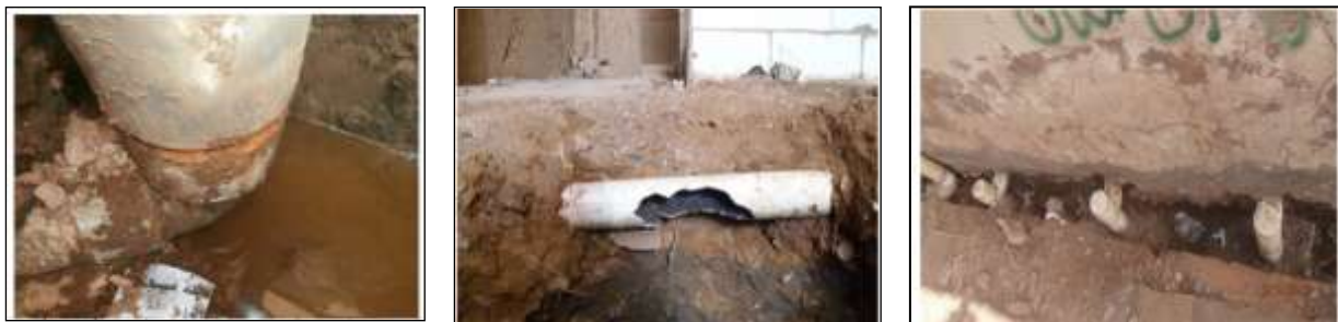
Figure.7 some pictures show cracks of drainage pipes leading to water leaking under the building
